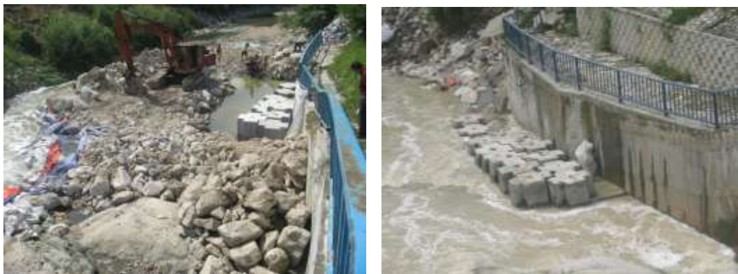
Figure 8: Example of Placement of VIP LINER (At Sg Kayu Ara, Damansara, P.J.)
