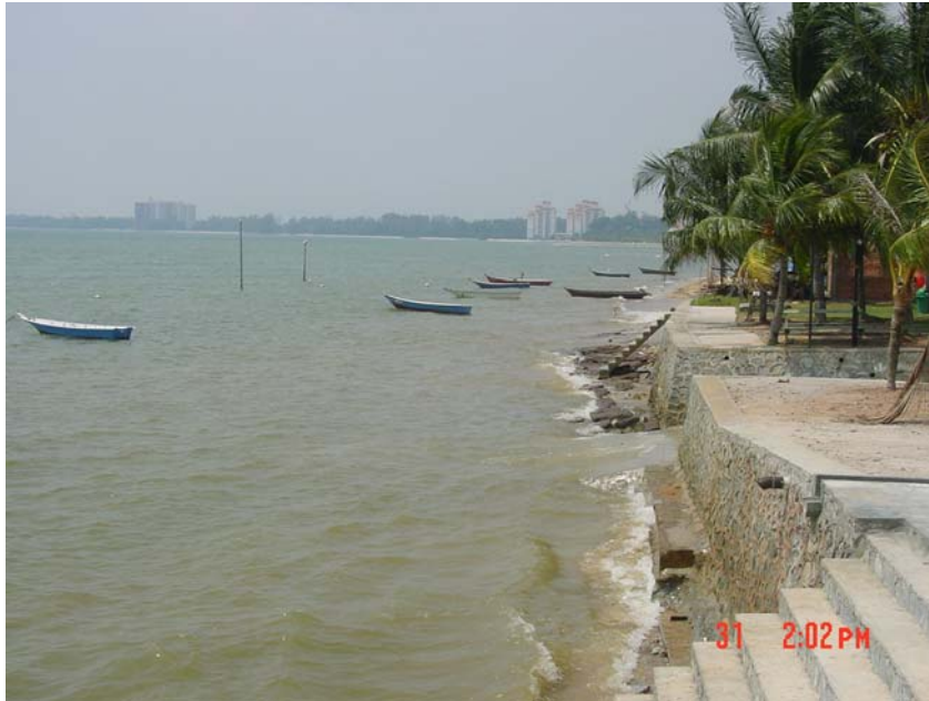
Figure 1: The vertical face of seawalls often enhance wave reflection and cause a lowering of the beach; Port Dickson.
