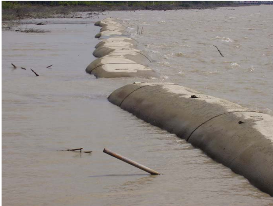
Figure 4: Sand-filled geotextile tubes used in Tanjung Piai, Johor to reduce wave energy on mangrove shoreline.
