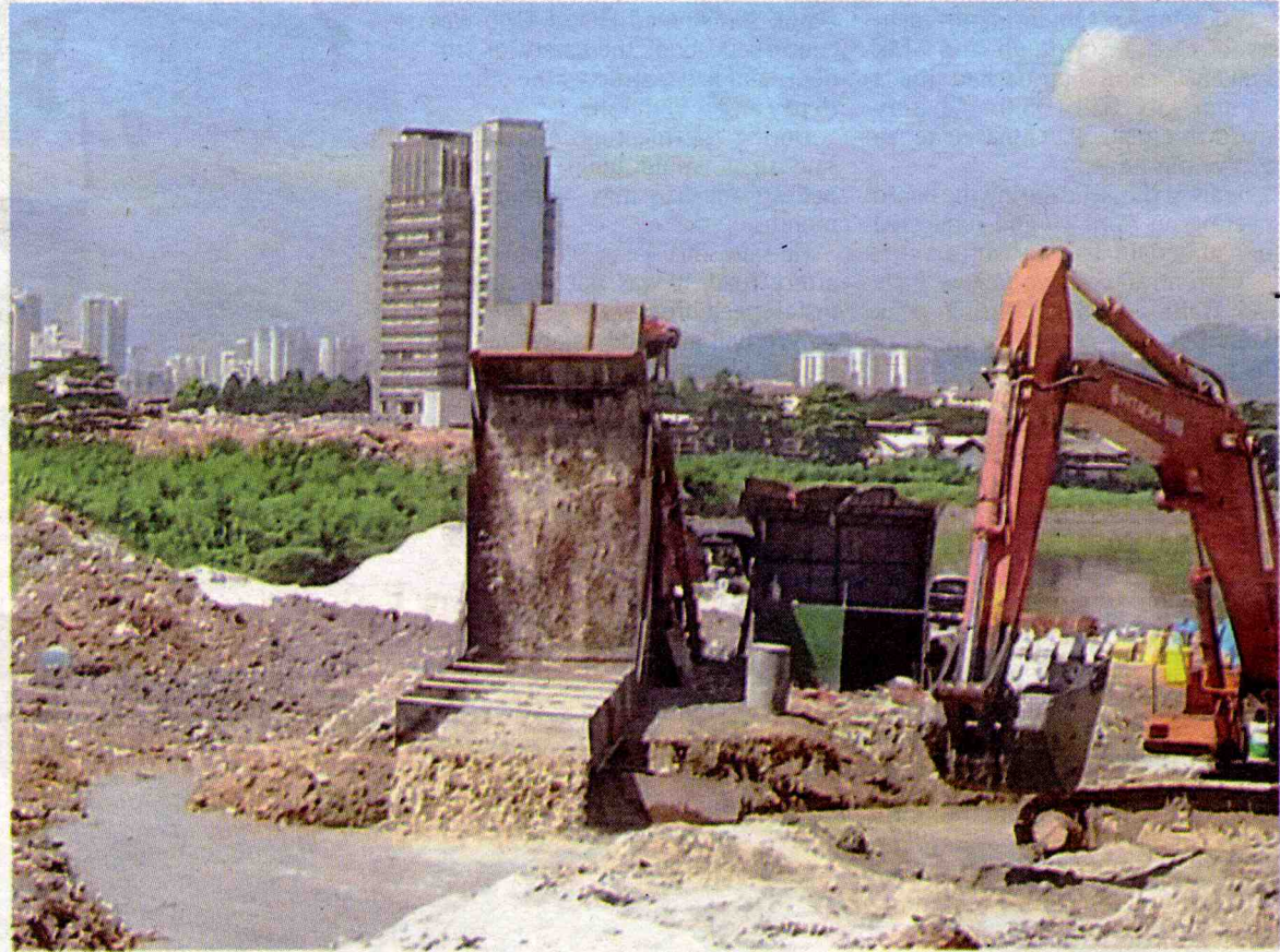
Concerned about their safety: Ongoing works by DID contractors at the Wahyu retention pond, which residents claim are sand mining activities.
