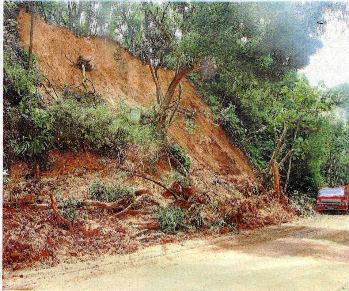
Coming down: A landslide in Jalan 5/64 in Bukit Gasing that occurred on Sunday afternoon after strong wind and rain hit several parts of Petaling Jaya.
