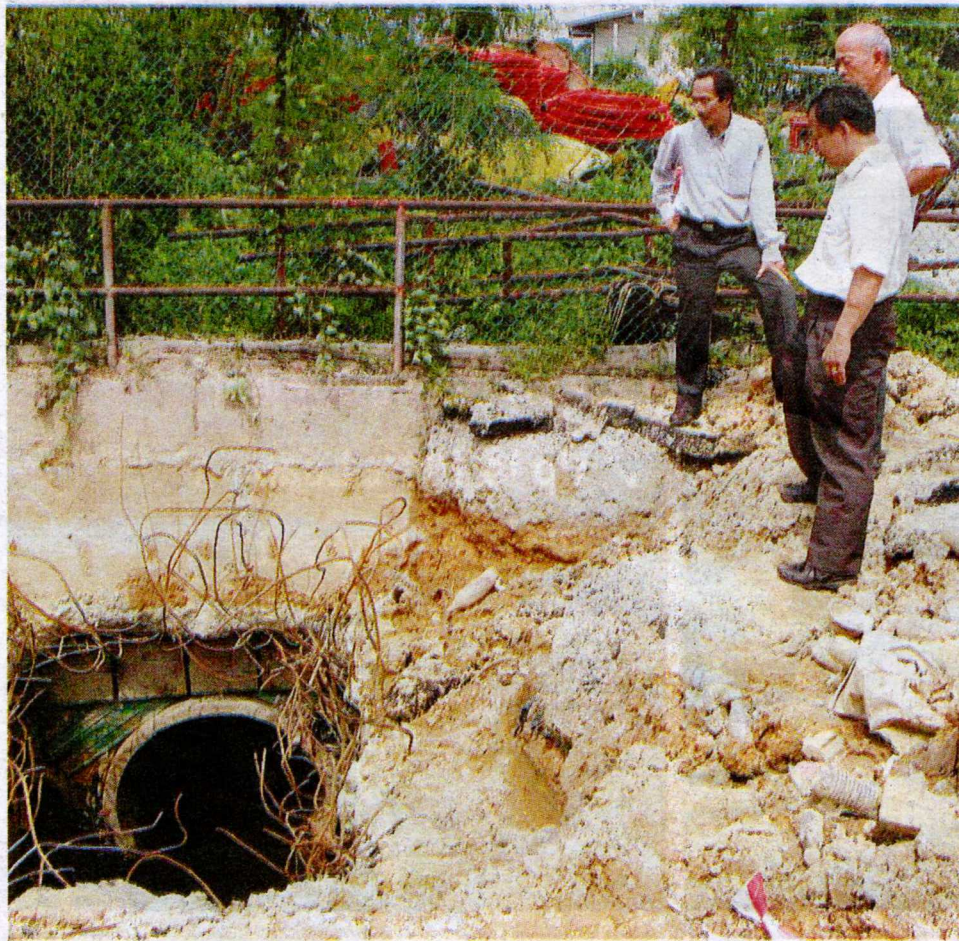
Yap (left) is joined by Cheng Hock Yew (second right) and Kuan Gan (right) as he inspects the works done by the contractors.
